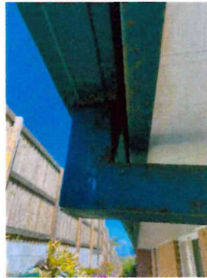
This downpipe on the NE corner of the garage is badly rusted and leaking. Persistent leaks are a conducive condition for termites.
